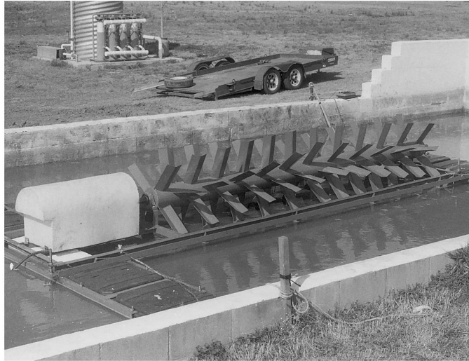
Fig. 4. A floating, electric paddle wheel aerator.
